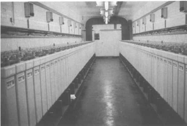
Fig. 3. View of one battery room at BEWAG's 14-MW h battery energy storage plant in West Berlin.
