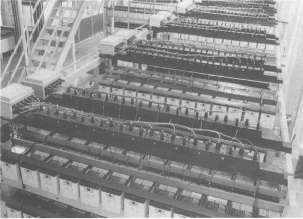
Fig. 6. View of battery rows at Delco's 600-kWh battery energy storage plant in Muncie.
