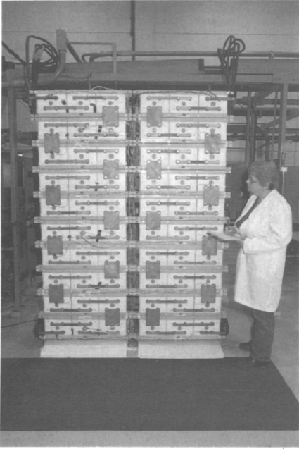
Fig. 8. View of GNB's sealed lead/acid battery under test at the BEST facility in Somerville.
