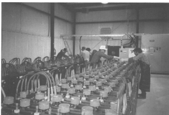
Fig. 5. View of battery energy storage plant at CEMC in Stateville.
